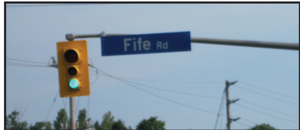
The street name sign on the pole is deficient because of diminished contrast (approaching 1:1) making it harder to read.
